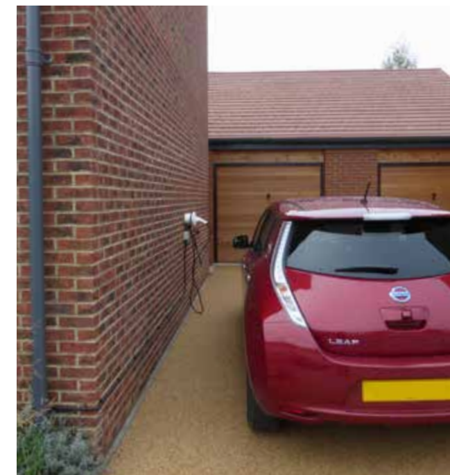
Home electric vehicle charging
